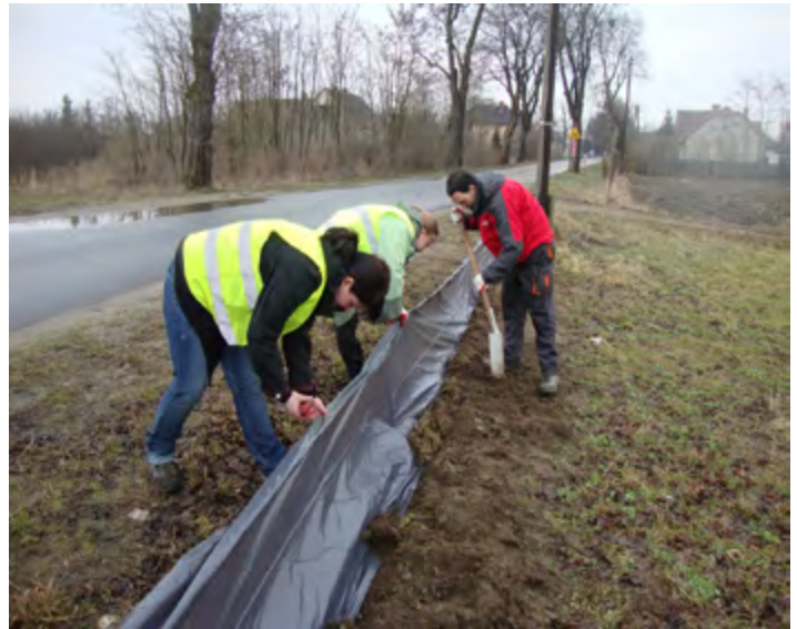
Installing the fencing along Lutycka Street in Poznan (Poland). Photo: Jan Kaczmarek.
