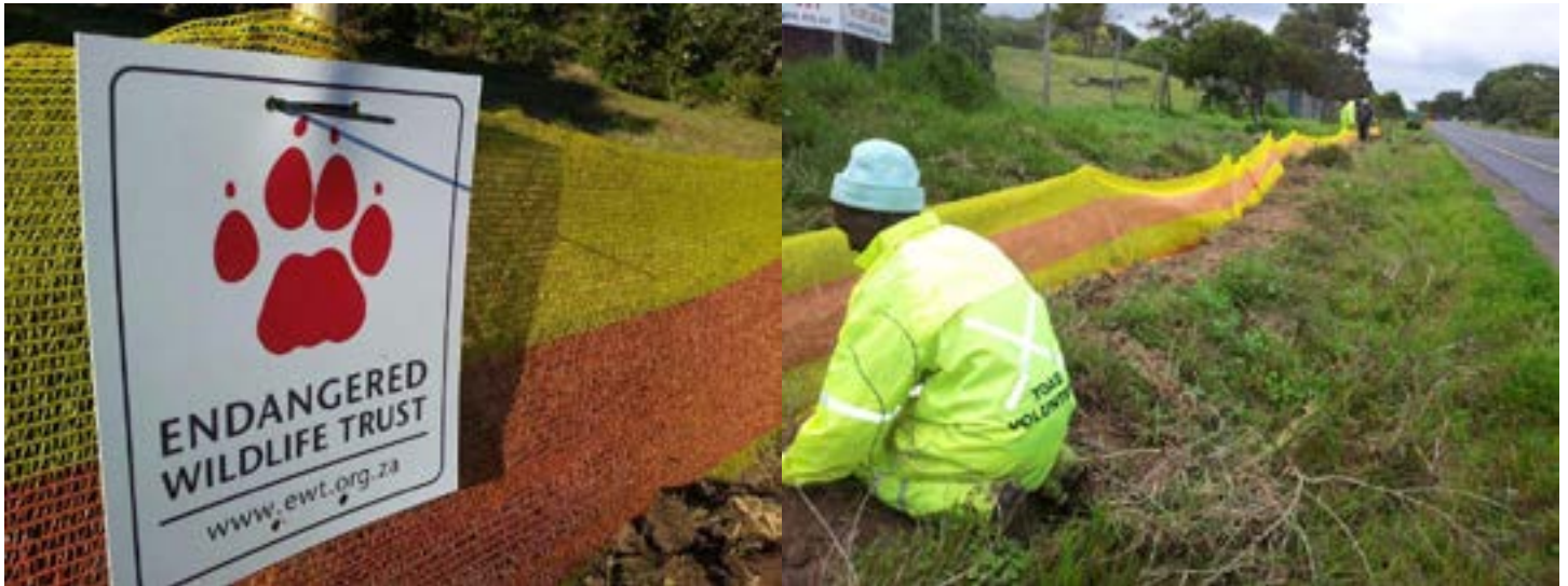
Barrier fencing erected along Noordhoek Road, Western Cape, South Africa. Photo: Alison Faraday.
